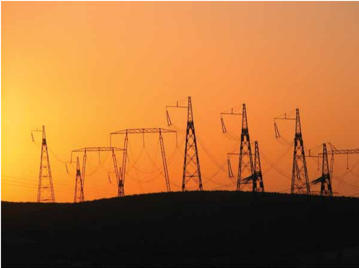
Power lines, Tajikistan.
