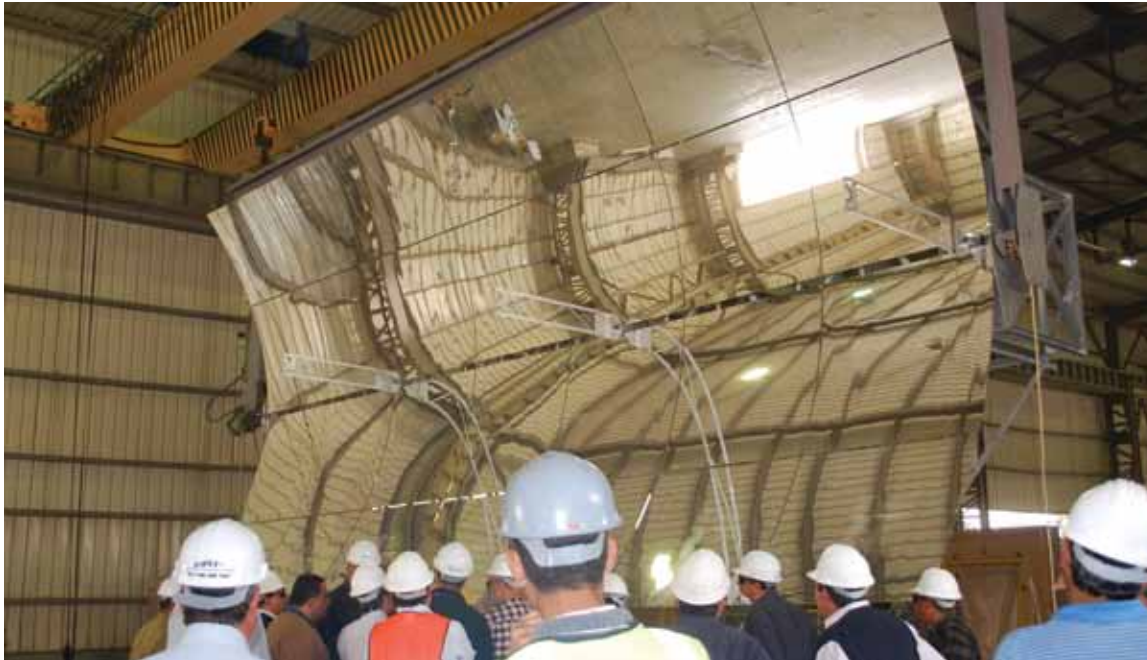
Parabolic trough reflectors for the WBG/GEF-financed Al-Kureimat solar thermal power plant in Egypt being assembled, March 2009.
