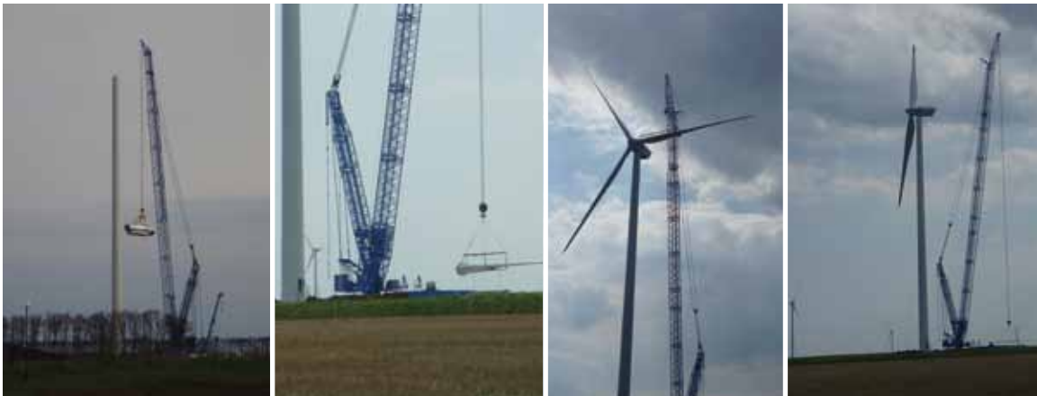
Construction of the 156 MW St. Nikola Wind Farm in the municipality of Kavarna, in the north-east of Bulgaria, on an elevated plain approximately 3km from the Black Sea (IFC project, "AES Kavarna"). The wind park comprises 52 3 MW V90 turbines, manufactured by Vestas A.S. (Vestas) of Denmark. The project includes a 33/110 kV substation, connected to the national grid through an 8 km transmission line.
